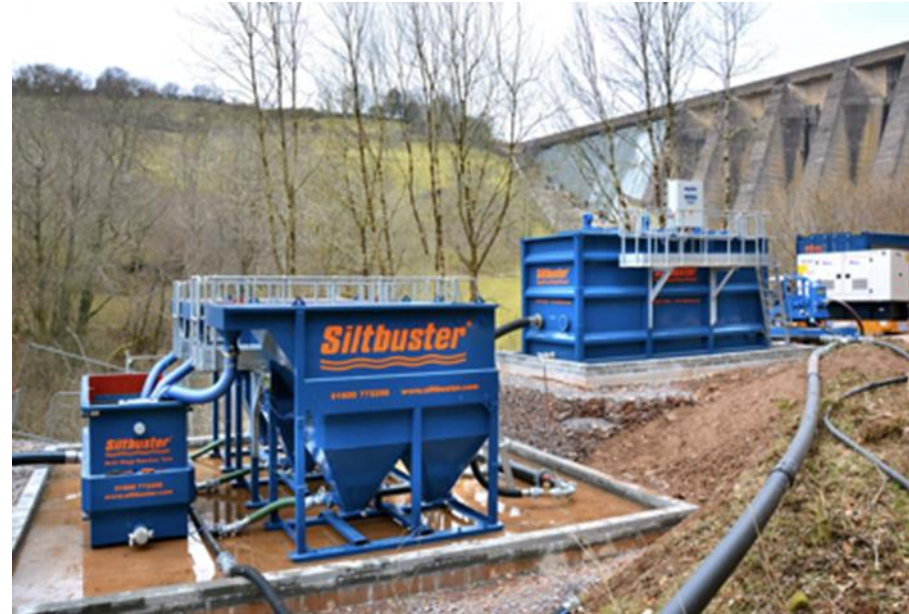
Chemical dosing / flocculation
